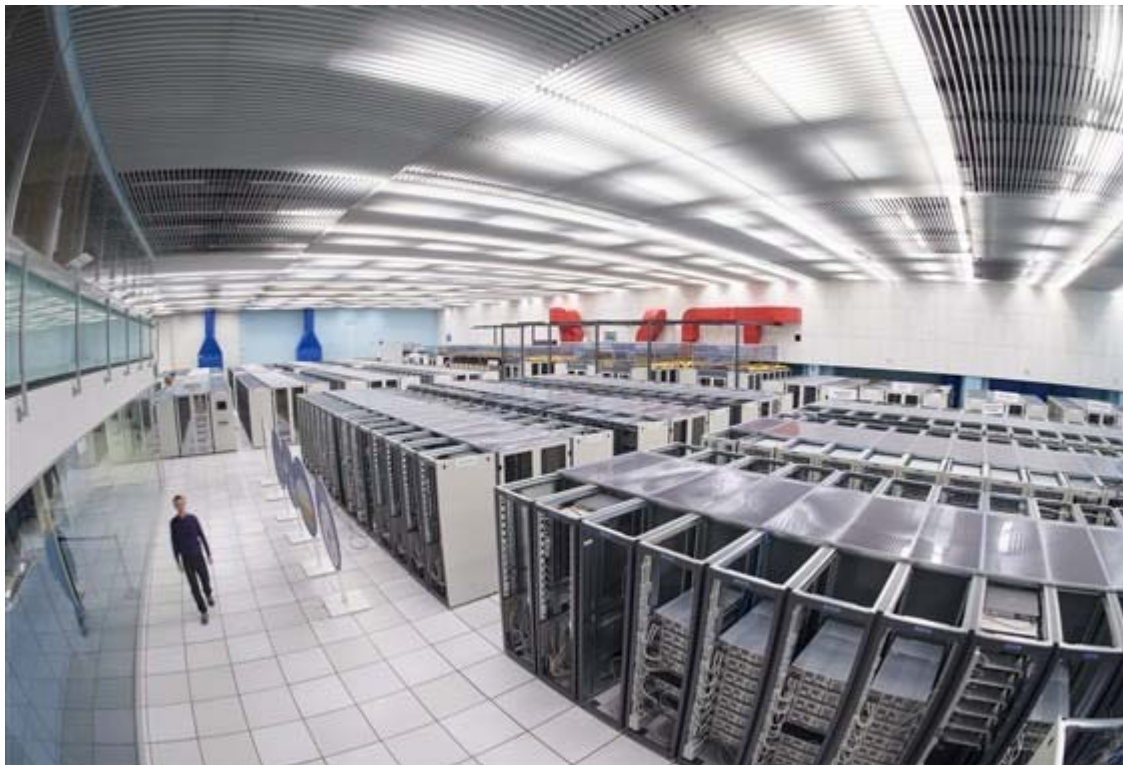
CERN's computer centre. Image: CERN
